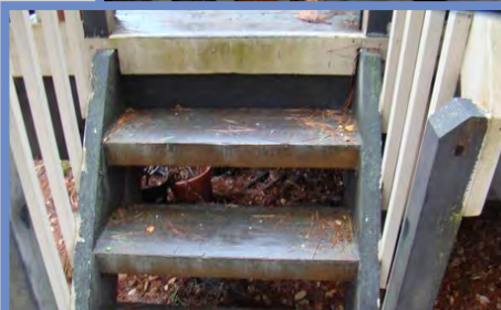
BEFORE - rotted stairs and deck
