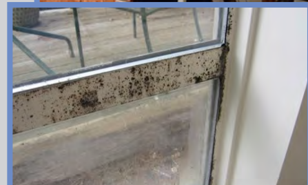
BEFORE - water damaged windows
