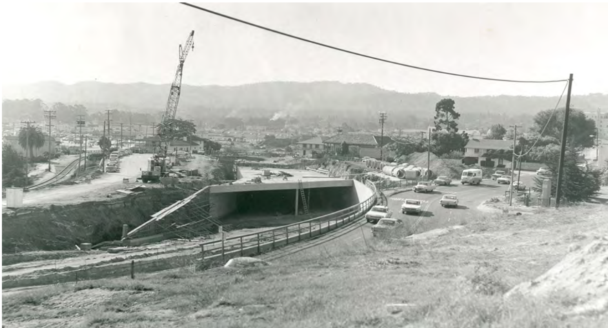
Figure 9-3. View of construction of Lighthouse Avenue Tunnel, looking south, August 28, 1967. The photograph shows Pacific Street traffic headed towards the Lighthouse Avenue curve at the Presidio (William L. Morgan, photographer, courtesy Monterey Public Library, California History Room).
