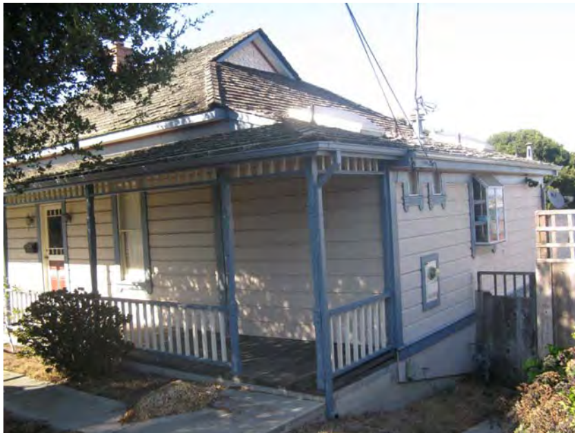
Detail of the primary and south facades from Pine Street (Page & Turnbull)
