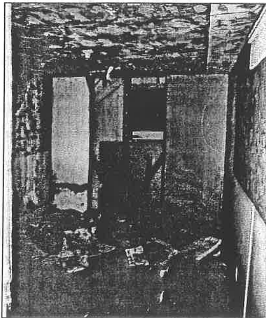
Figure 9: Another interior view showing the deterioration of a typical room.
