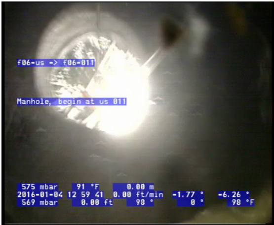
Photo: 4_1A, VCR No.: aguajito sewer spill 0FT, Upstream Manhole, Survey Begins
