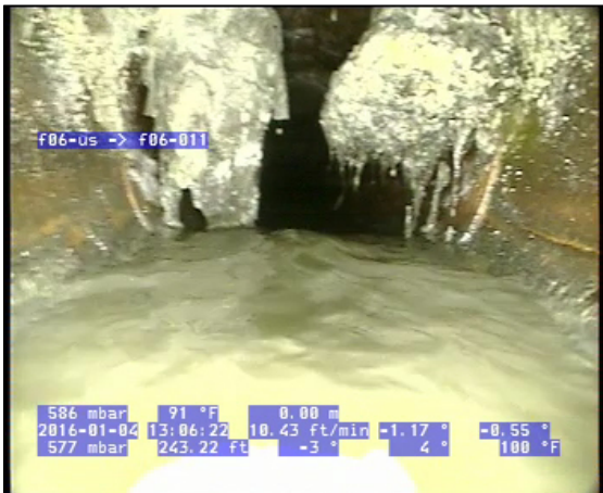
Photo: 4_3A, VCR No.: aguajito sewer spill 244FT, Roots Medium Joint, from 09 to 03 o'clock, 25 %, within 8 inches of joint: YESR
