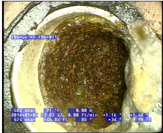
Photo: 4_2A, VCR No.: aguajito sewer spill 145.8FT, Tap Saddle Active, at 02 o'clock, 4", within 8 inches of joint: NO
